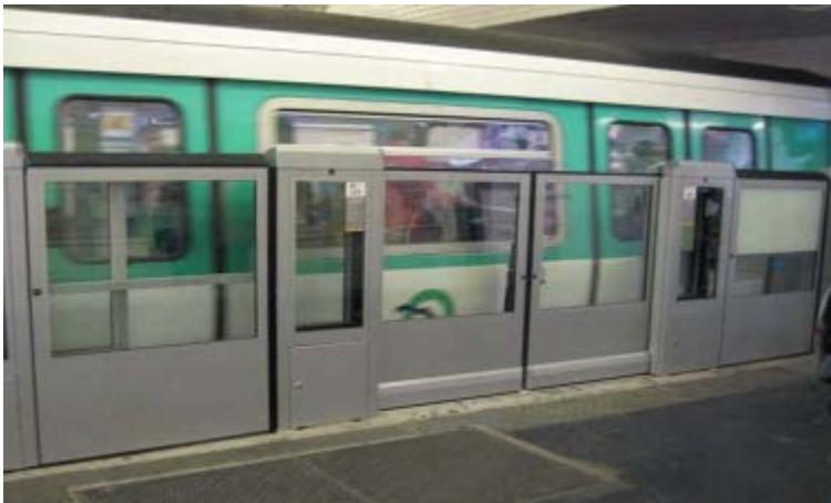
Figure 33: Platform screen door
